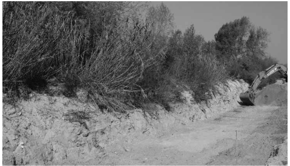
Arundo donax is being unintentionally spread by this backhoe. Simple measures can be taken to prevent mechanical dispersal of arundo.
